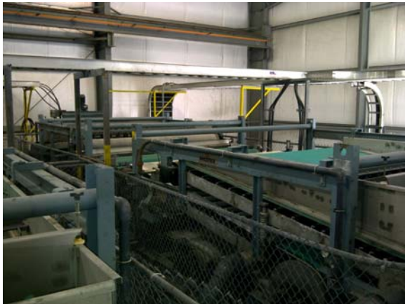
Figure 3: Belt Presses in the Press Building
