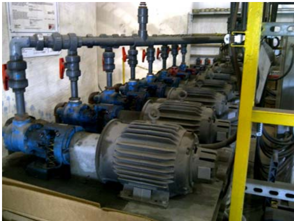
Figure 7: Eight Pumps for Coagulant
