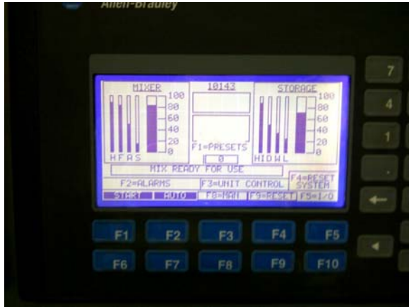
Figure 5: Control Panel - Anionic Flocculant
