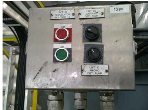
Figure 8: Flocculant Manual Control Box
